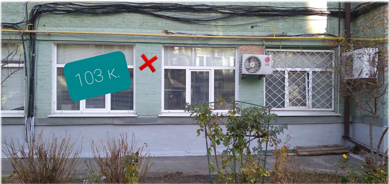
Room 103 (Server Room) – Place of AC external unit installation, street view
